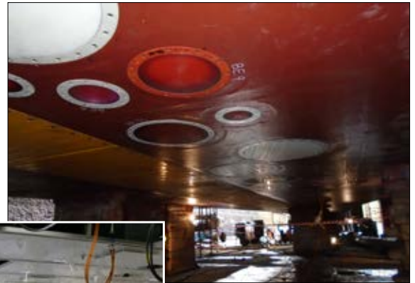
The acoustic sensors within the bottom of the vessel
